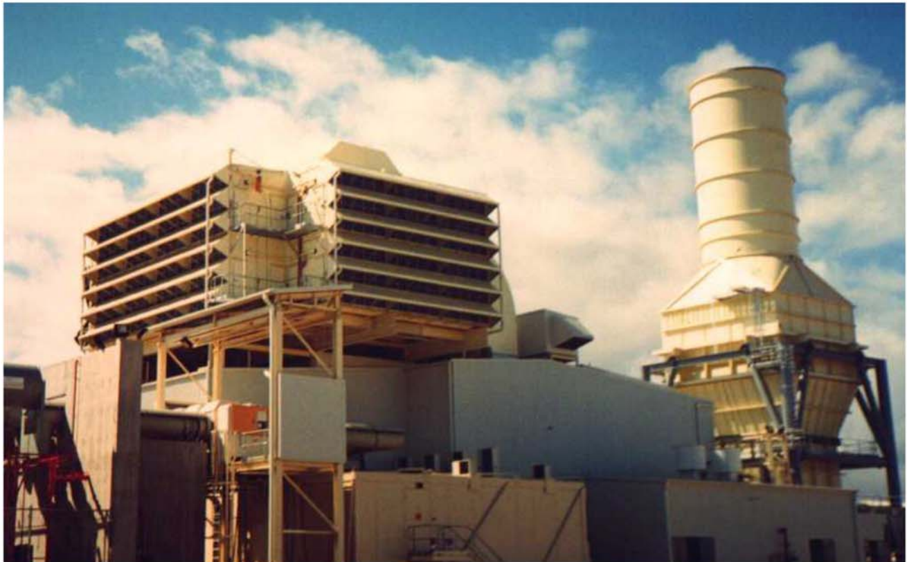
Gas Turbine Enclosure
